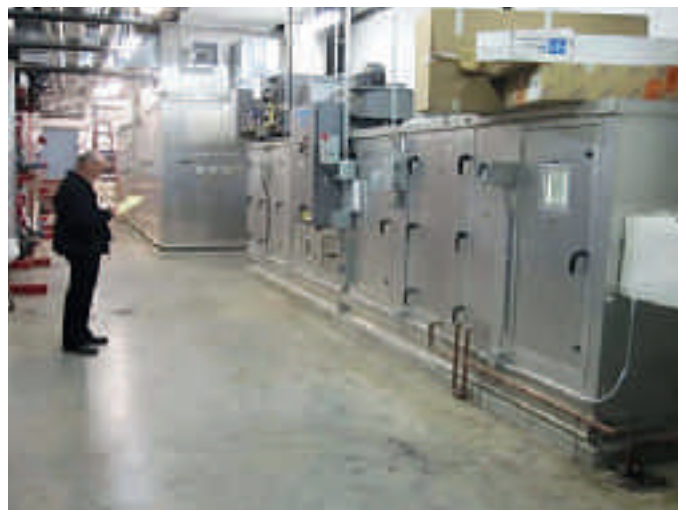
3. One of the AHUs at the Library Annex at Cornell University. Project partner Peter Herzog of Herzog/Wheeler & Associates is shown.
