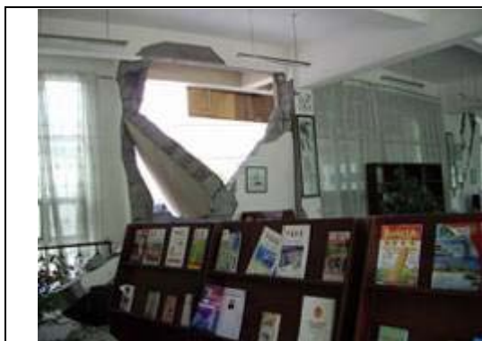
Pic.29 The destroyed library
