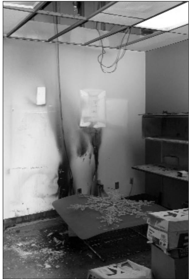
An interior office with evidence of smoke damage on the walls.
