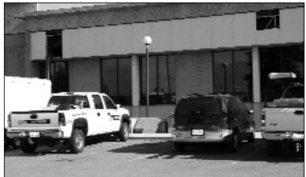
South side of the Sevier County Records Office showing roof construction; welding occurring in the building's attic caused the fire.
